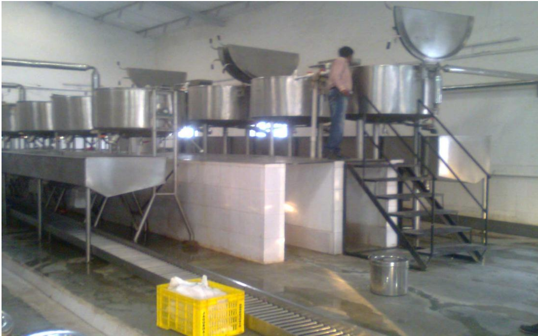
Centralize kitchen: Equipped with modern machinery for preparing the food
